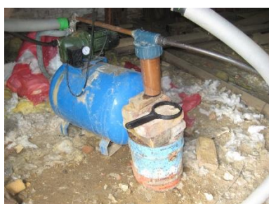
Water supply with inadequate filtration system
