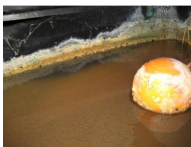
Uncovered storage tank
